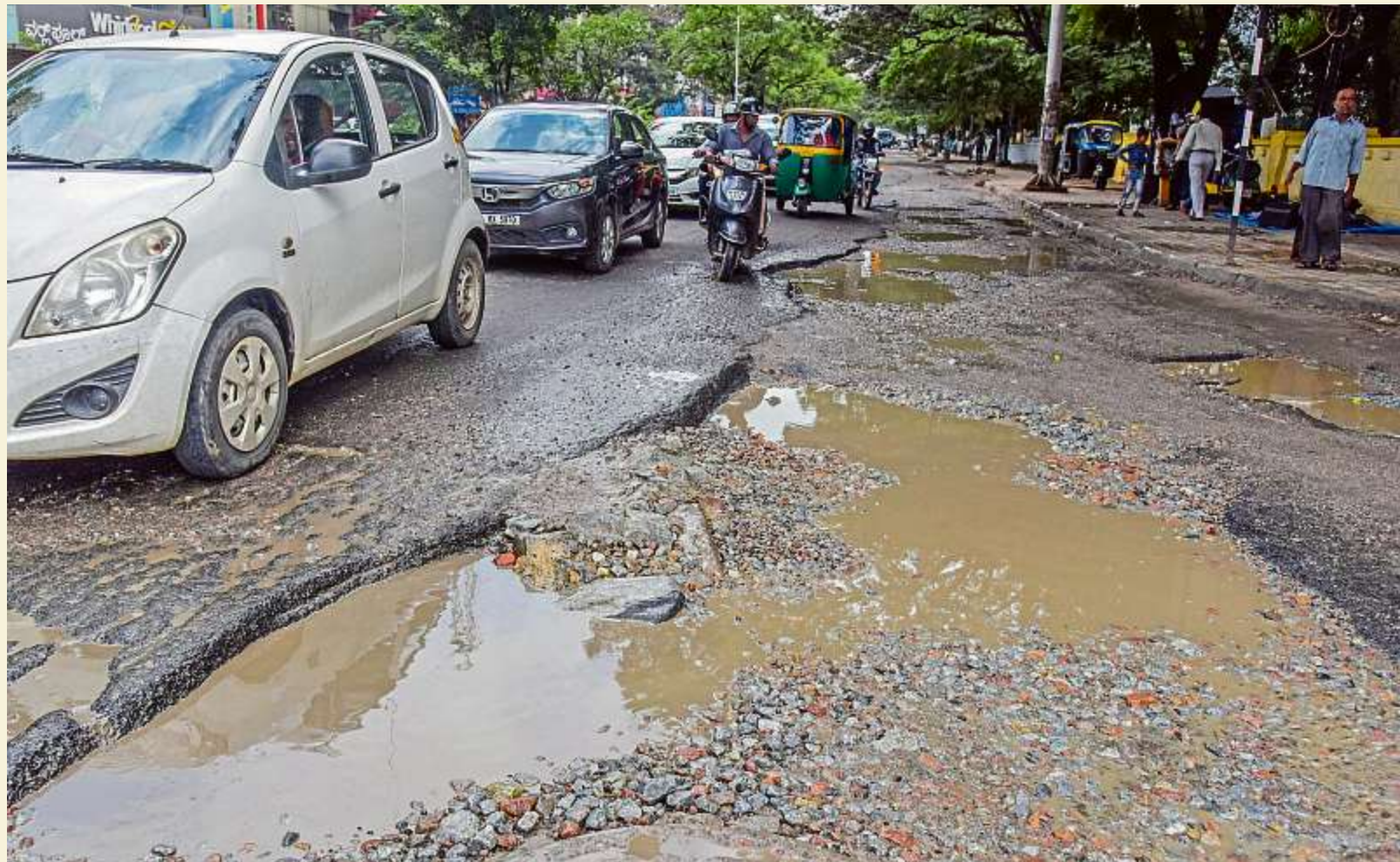
KH ROAD The potholes are getting deeper and bigger on this arterial road, near the KSRTC head office and Shantinagar bus terminal. Thousands of vehicles use this stretch, and no one is doing a thing about the hazards. DH PHOTOS BY SK DINESH AND PUSHKAR
