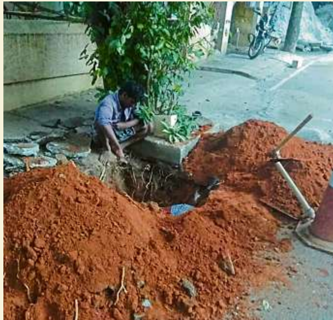
JAYANAGAR Private companies are digging up roads to lay cables and, in this case, instal poles.
