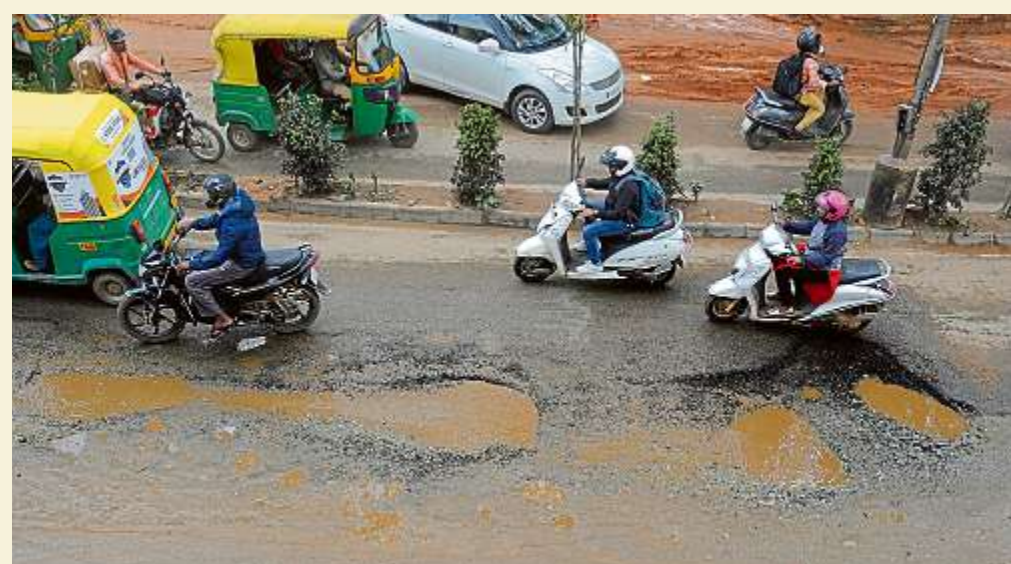
THANISANDRA MAIN ROAD The potholes here are deadly. Poor maintenance of roads is among the major causes of non-fatal accidents, says traffic police. DH PHOTO BY PUSHKAR V
