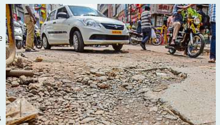
BVK IYENGAR ROAD: This is one of busiest streets for business, and it is in pathetic shape. Potholes force motorists to stop, swerve, and often trigger accidents.
